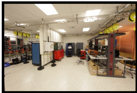
Distribution Automation Lab
